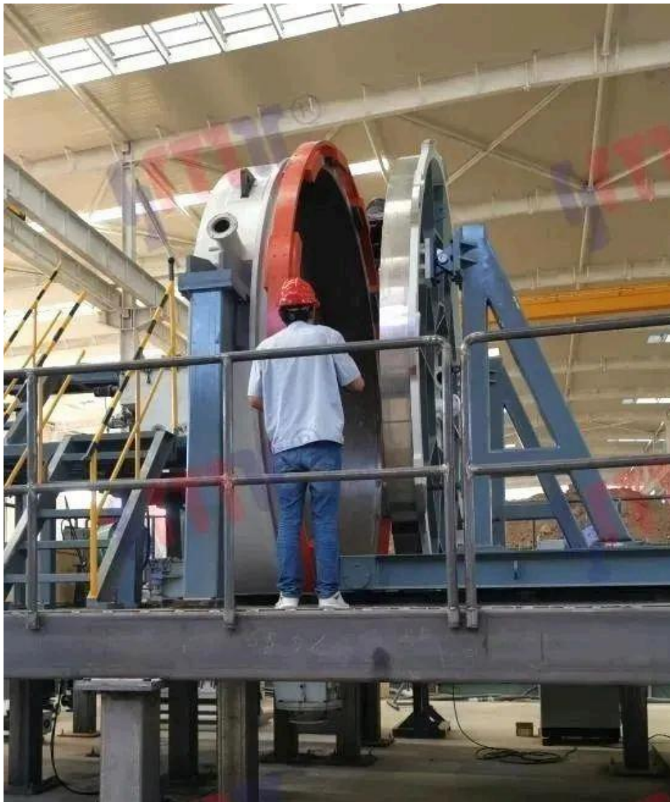
△国产SS-PREP®粉末制备设备安装调试
