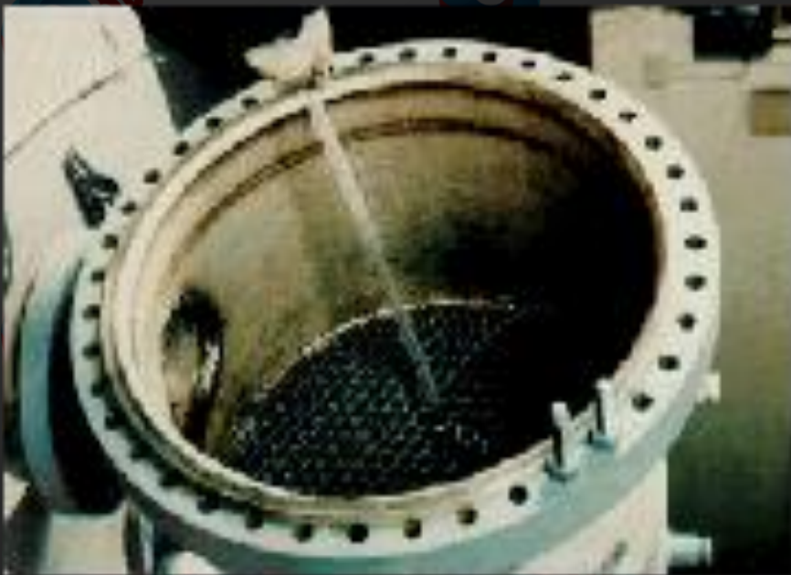
Under-performing, 324 tube, heat exchanger
